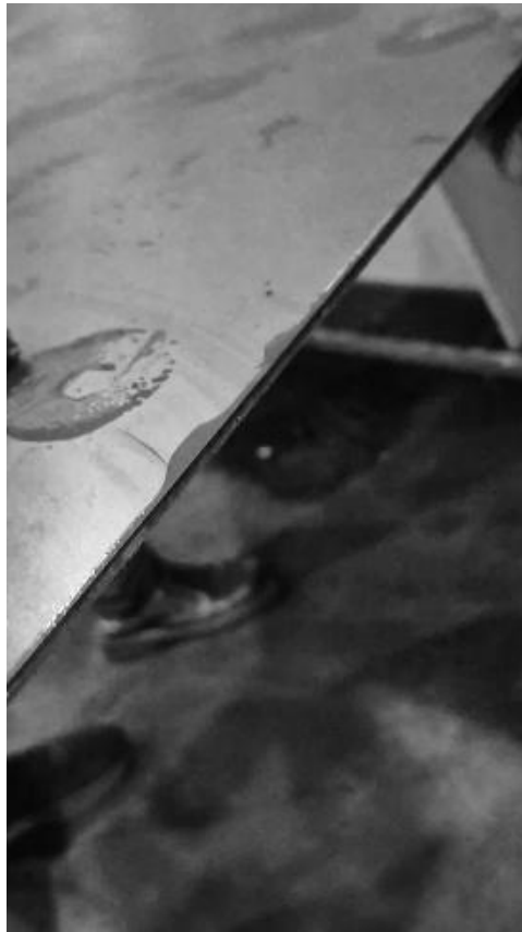
Figure 2. Pre-retrofit cutting condition on a 6 mm steel plate
