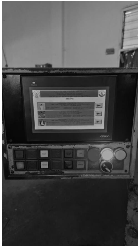
Figure 15. Control panel with selector, push buttons, and indicators
