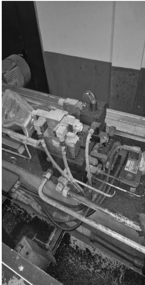
Figure 3. Solenoid components identified during troubleshooting
